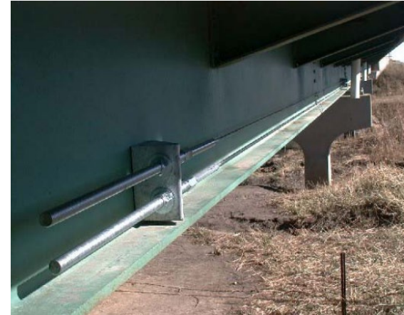
Steel Girder Bridge located in Guthrie County, Iowa: CFRP (P-T) Rods
