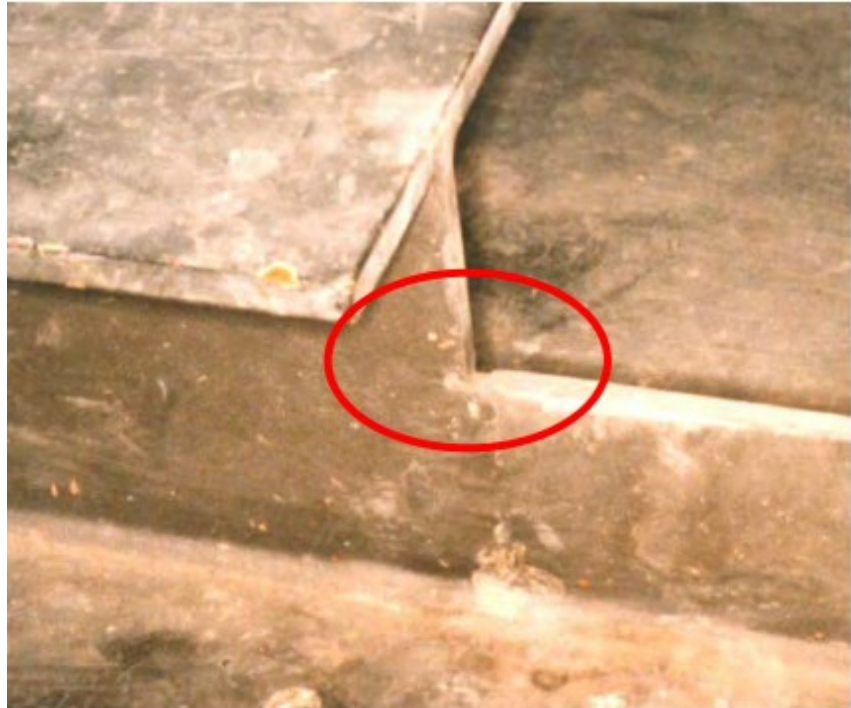
Bad coped beam detail (sharp corner)
